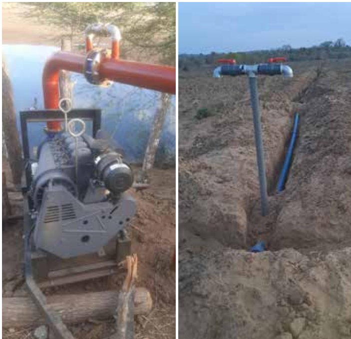
Matata Irrigation Scheme has been established with a pump and piping installed. The 60 community beneficiaries will plant their first seeds in the new year
